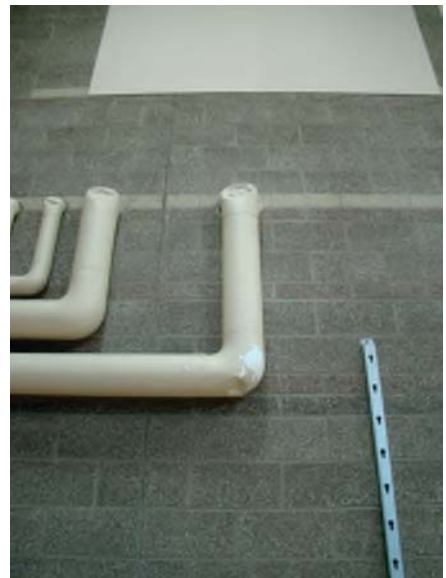
Figure B20.4 – Damaged Duct
