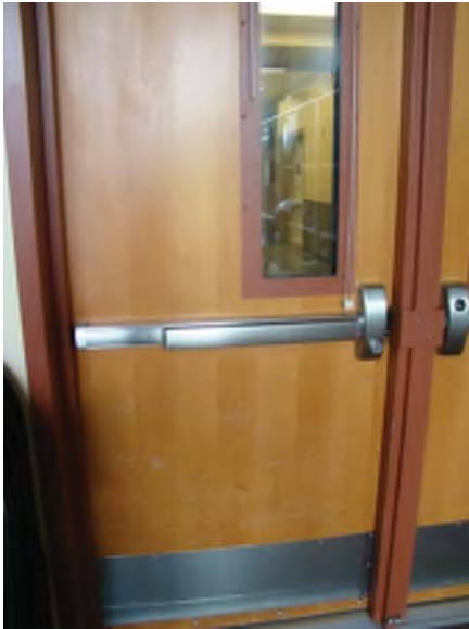
Figure B30.2 – Worn Doors
